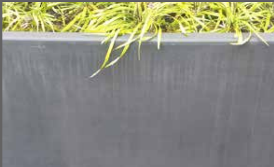
Fibreglass planter after 5 years before treatment
